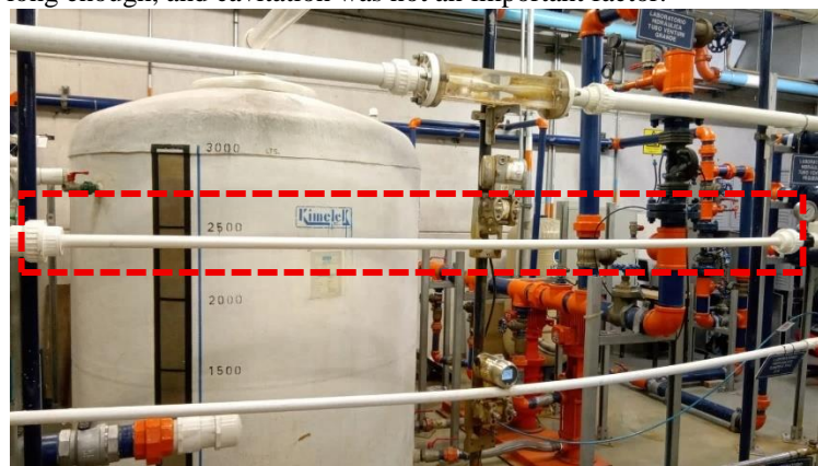
Figure 13. In the intermittent it is the pipe (1/2" diameter PVC) that could be changed for the model
